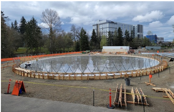
Chilled water storage project behind the Central Power Station
