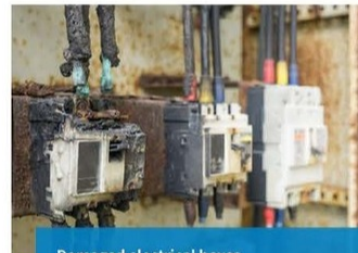
Damaged electrical boxes.
